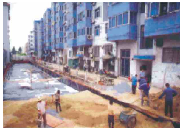
October 2003: The vertical flow constructed wetland was settled into the channel. The first construction period was designed for a daily load of 80 m 3 . The extension of 600 m 3 per day is provided.
