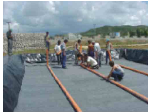
Drainage system on the filter ground. Albania Draht SH.P.K., Vorë, Albania (60 employees)
